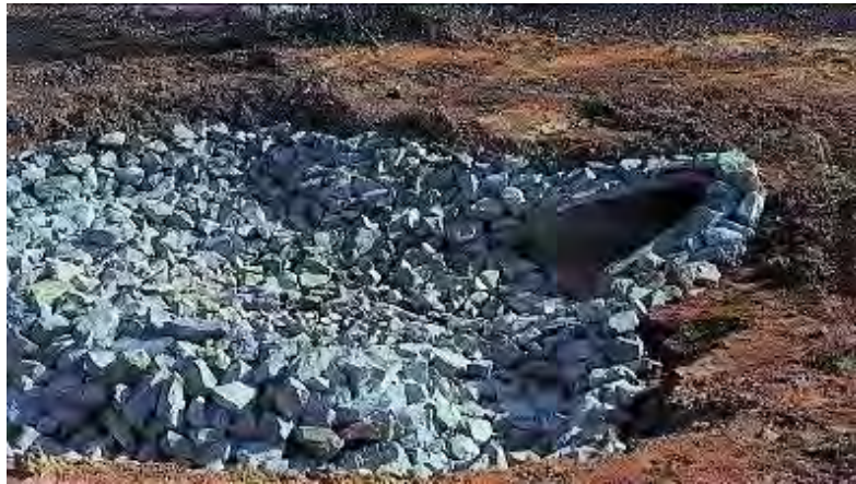
Rip-rap used for energy dissipation at outfall
